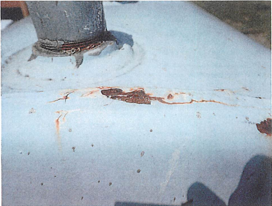
Photo 9: Coating failures and surface rust on the top of the tank
