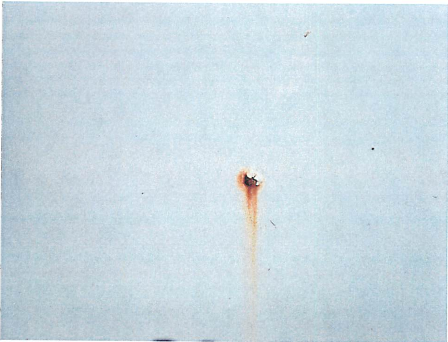
Photo 6: Exterior sidewall impact area with surface rust
