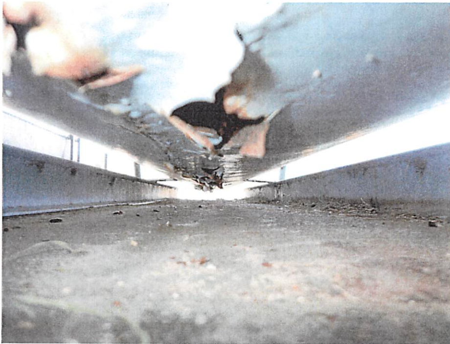
Photo 12: Coating failures and surface rust on the underside of the tank
