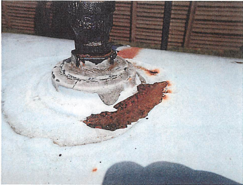
Photo 10: Coating failures and surface rust on the top of the tank at the penetration area
