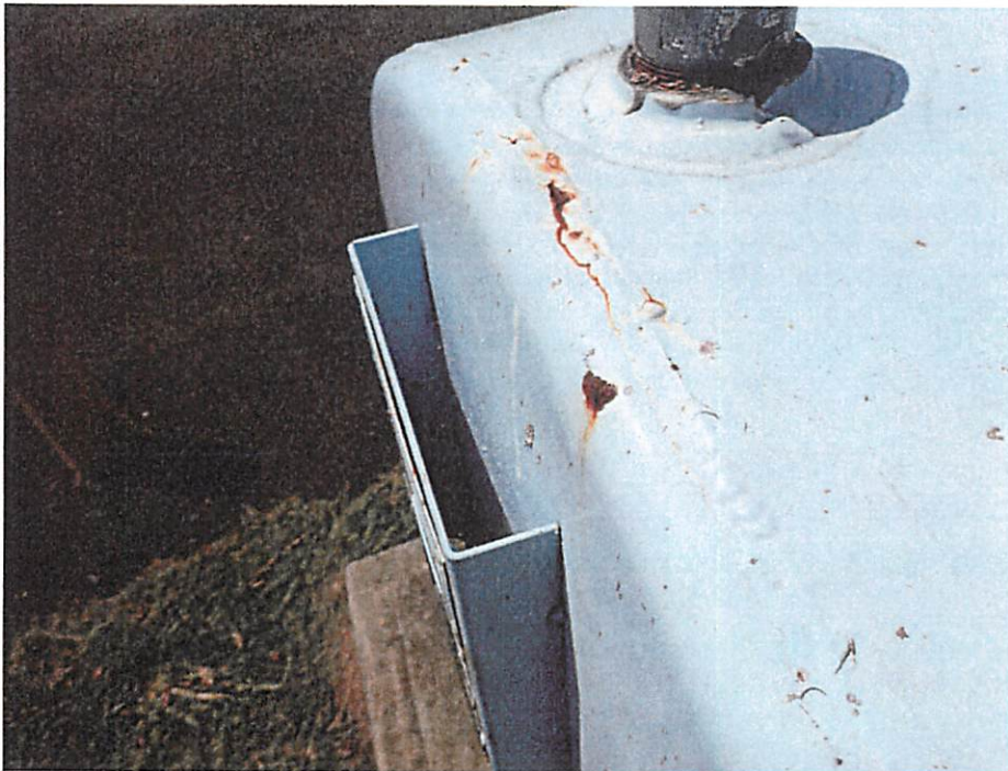
Photo 8: Coating failures and surface rust on the top of the tank
